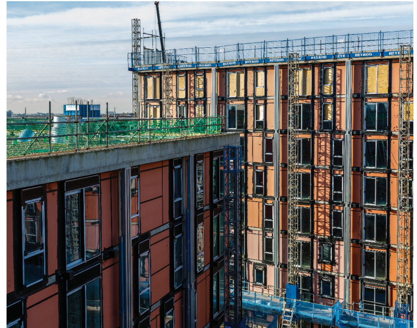
Knauf Windliner installed on Middlewood Locks mixed-use development in Salford, Greater Manchester
